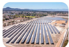
Atlantis solar PV plant
